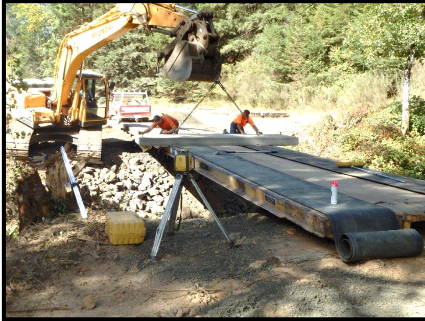
A livestock/farm bridge being installed across Mehl Creek. This bridge will enable the landowner to move livestock and equipment across the creek without having to enter the creek.
