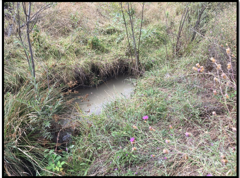
Photo 3. Drainage between Highway 42 and McDonalds.
