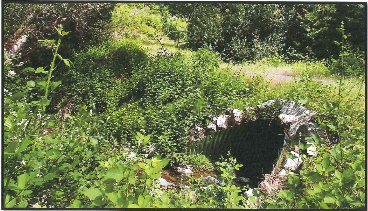
Briggs Culvert Inlet Post-project June 2015. The site is stable and passing all fish.
