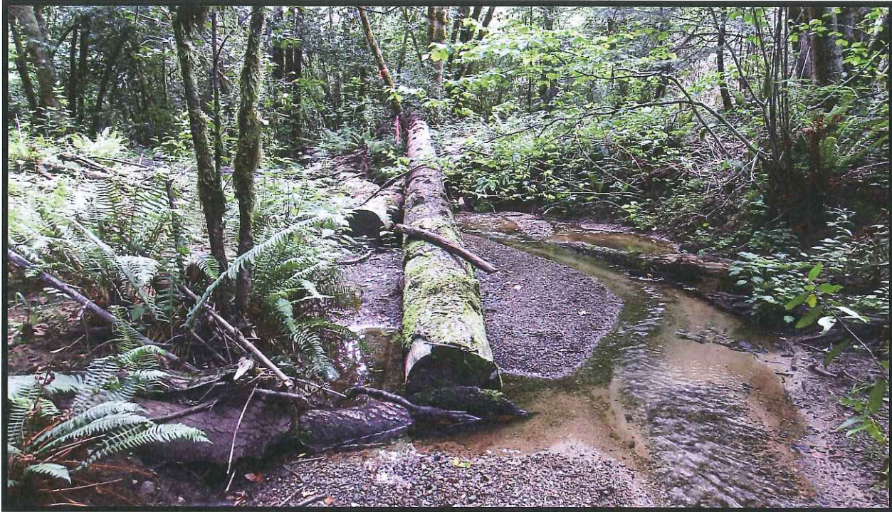
Site #15 Briggs Property Post-project June 2015. Laying large materials in the creek created meanders, islands, side channels, and deeper pools.
