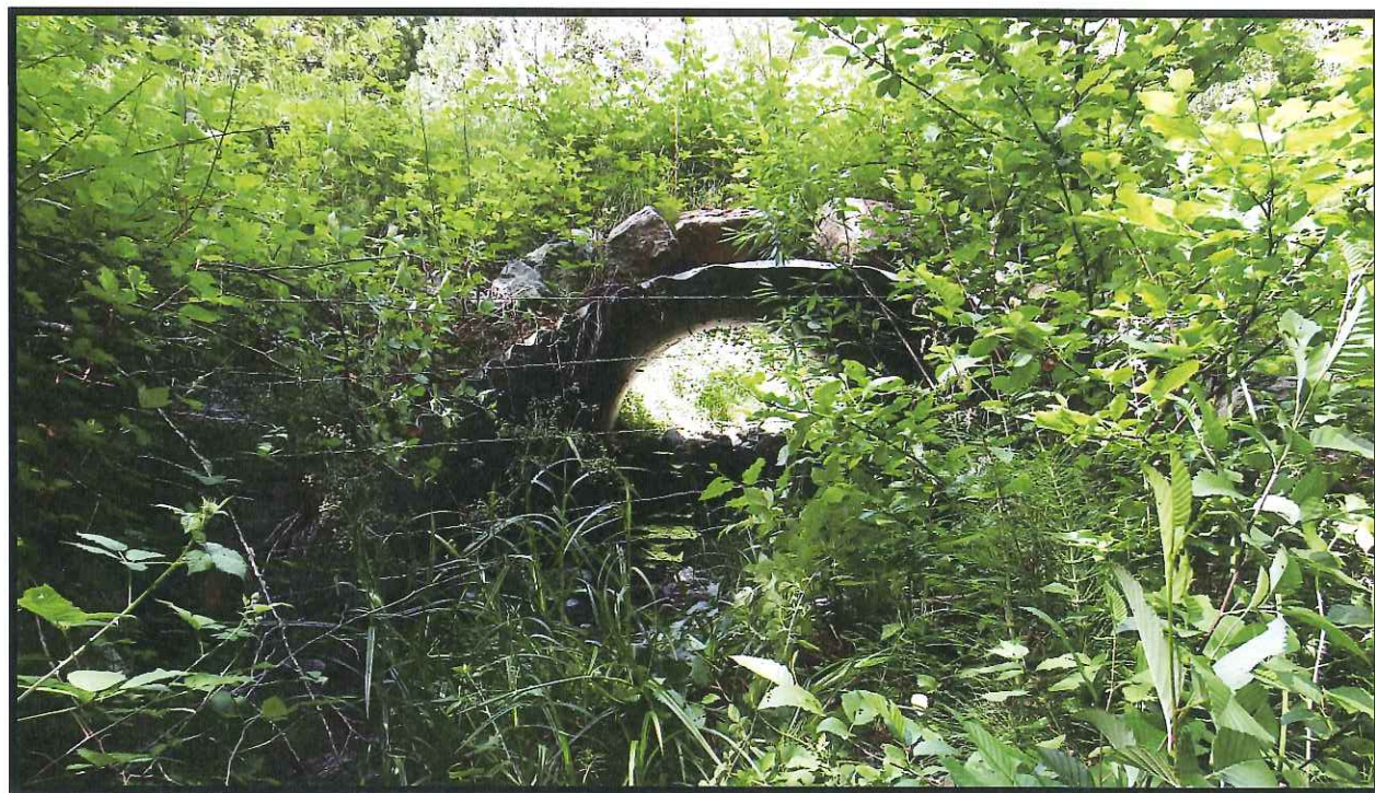
Briggs Culvert Outlet Post-project June 2015. Vegetation, including small alders, have vegetated all the disturbed areas around the culvert replacement.
