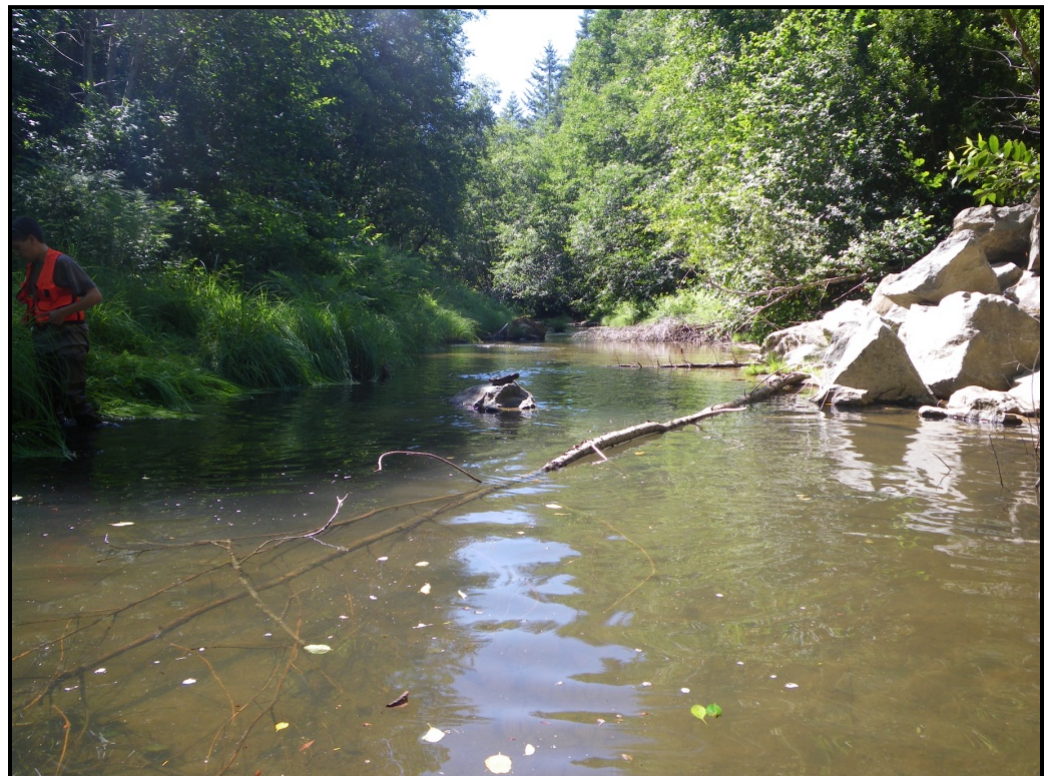
Photo #26: 7/2/09 prior to boulder placement boulders staged at right of photo Looking upstream
