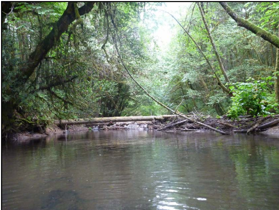
Photo #10: Weir #8 More debris accumulation 7/12/2011 Looking downstream at weir
